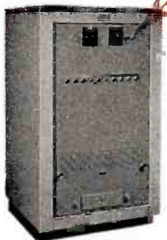
COMPLETE TRANS- MITTER CONTROL IN UNDER-WINDOW CABINET
